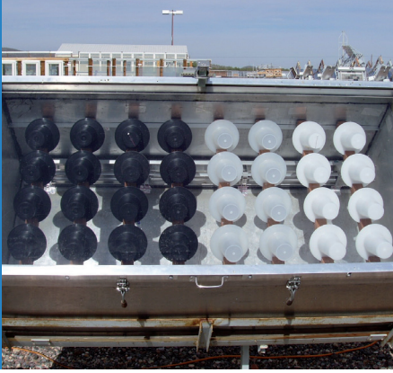
Instrument panel / door panel box in Arizona (Photo: ATLAS MTT).
